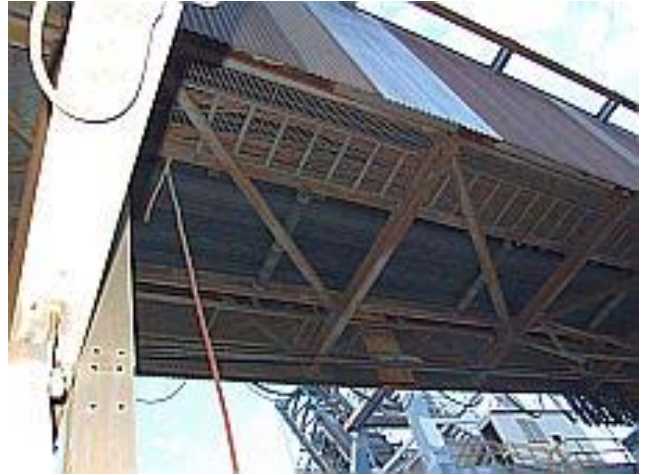
Figure 1.18 Up view of conveyor 3
