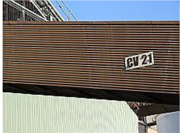
Figure 1.7 External view of conveyor 21
