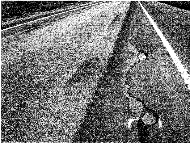
York to Quairading Road “Upgrades” after less than 3 months.
