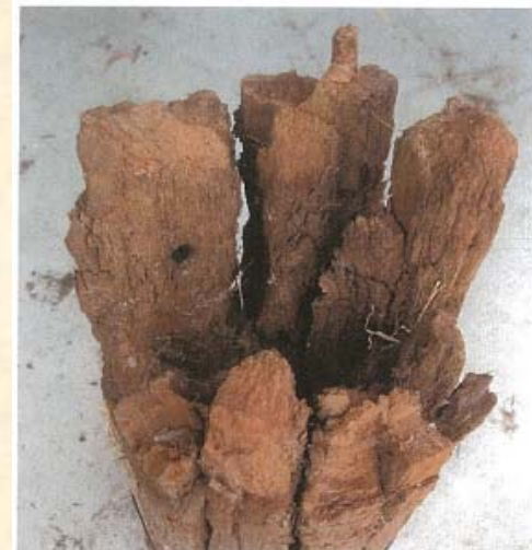
Picture 5. Pole PID# 338952 showing extensive decay and missing timber
