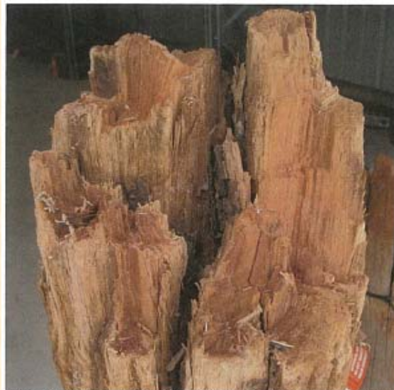
Picture 3. Pole PID# 338950 showing rot and brittle failure in the cross section
