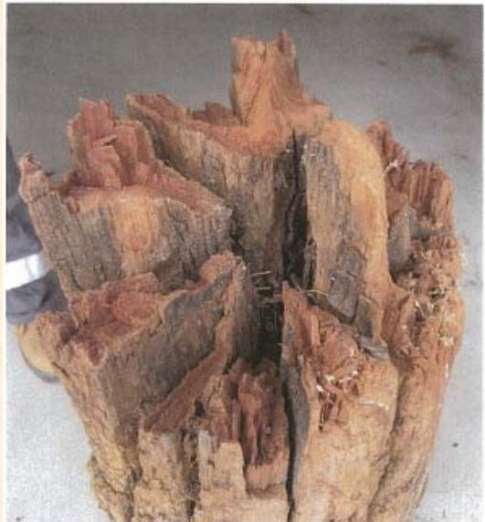
Picture 2. Pole PID# 338949 showing severe rot in the cross section and
