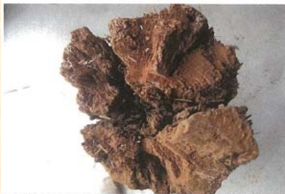
Picture 4. Pole PID# 338950 showing wide cracks in the radial profile and brittle
